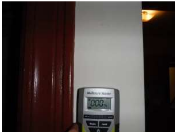
Figure 20 Random checking on inner wall where dry.
