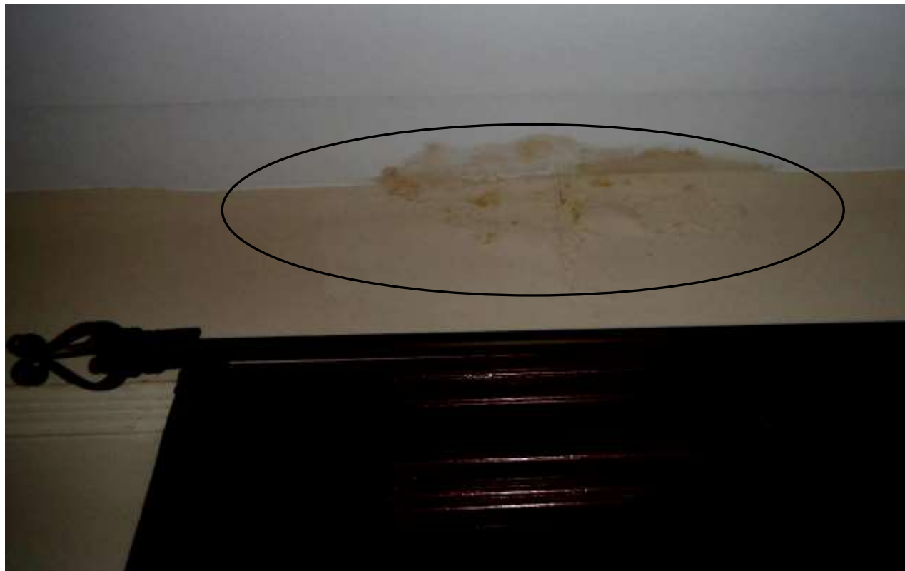
Figure 24 Flakes paint around ceiling water stains/leak; see roofing section comments.
