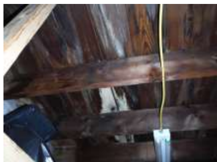
Figure 15 Water stains on roof sheathing.
