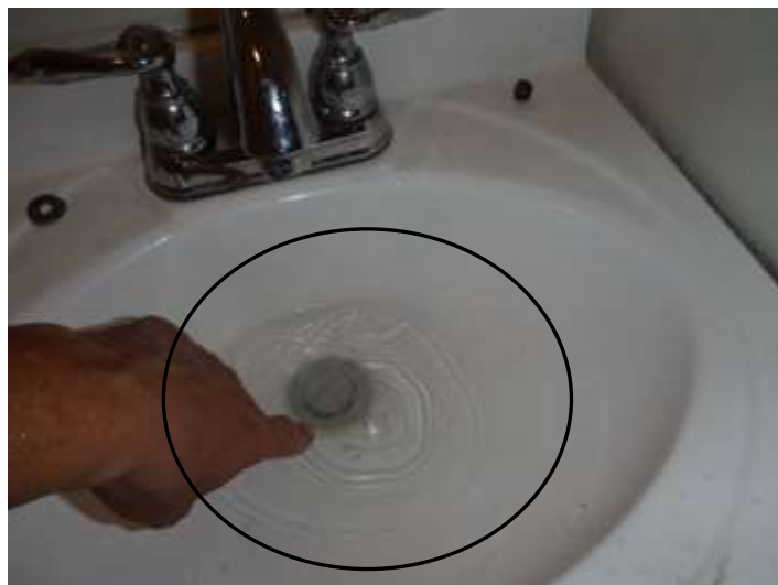
Figure 19 Have plumber evaluate slow drainage in building; see plumbing section comments.
