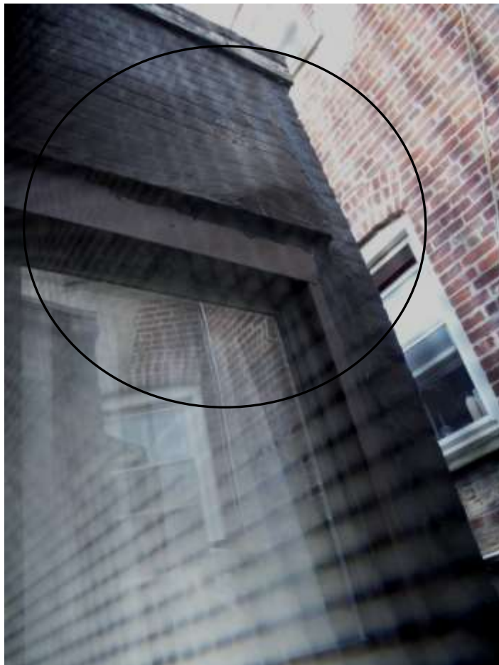
Figure 13 Buckled siding and tarred window & brick; view from apartment bathroom window. Right side of main building was inaccessible.
