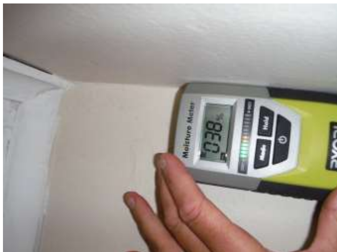
Figure 18 Active moisture detected in apartment rooms, closets and hallway.
