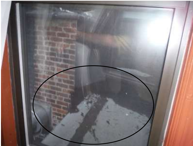
Figure 4 Poor roof conditions; lower main roof (view from apartment window).
