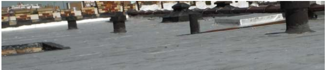
Figure 3 Tarred over roof penetrations; unconventional handyman.
