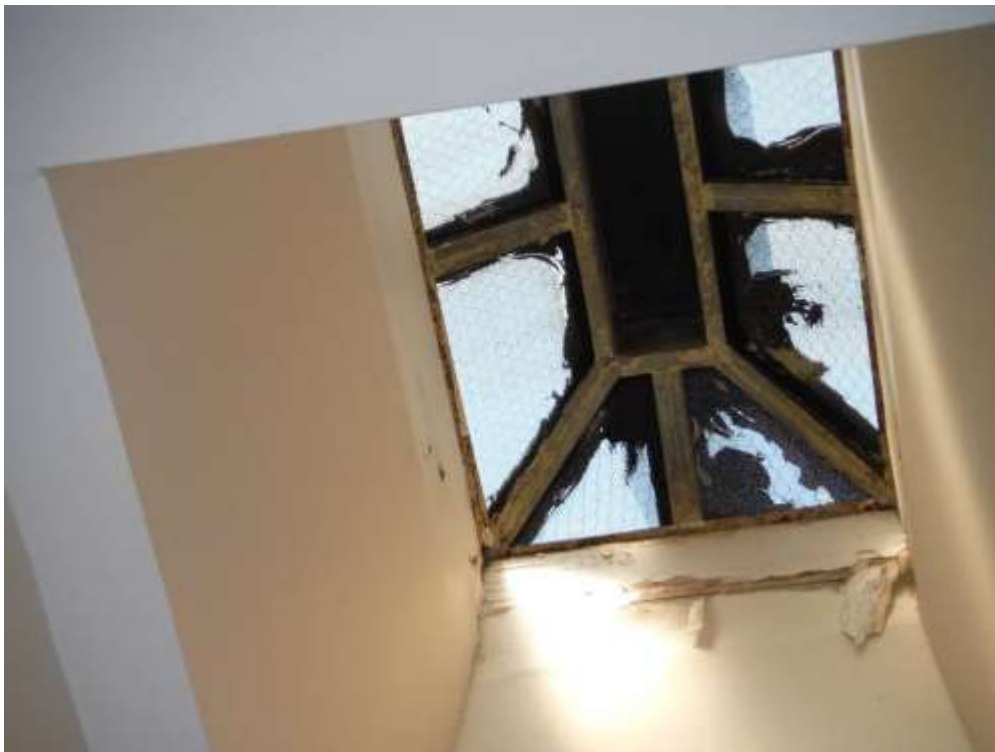
Figure 5 Tarred skylight. flaked paint, water stains; have roofer evaluate along with roof.
