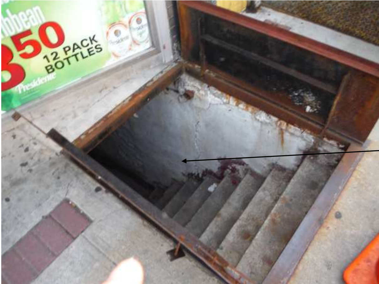
Figure 1 Dangerous; fall hazard to basement when door is left open. Follow-up with a safety supply company & consultant for railings, fencing and conveyor when receiving shipments or products for basement storage.
