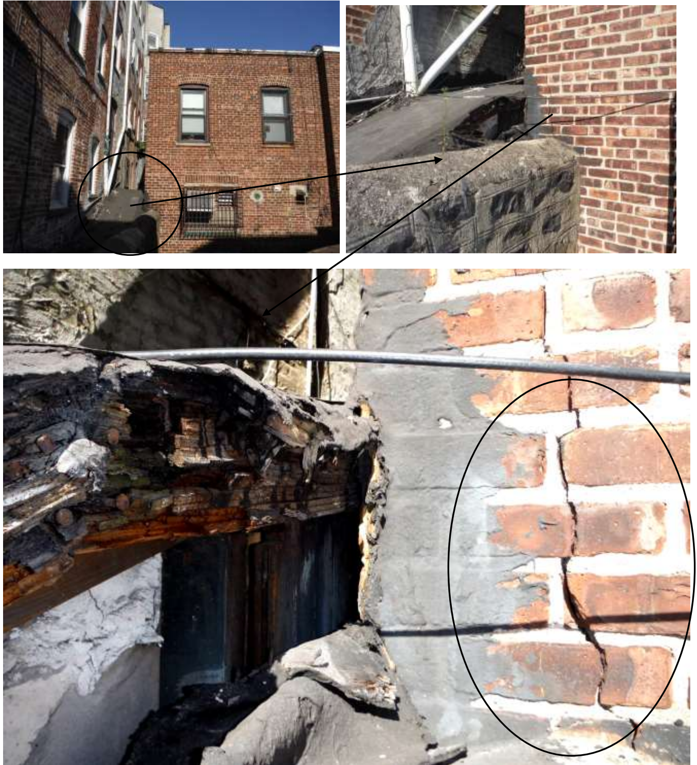
Figure 11 Structural cracks, rot on adjacent shed roof between buildings. Water entering cracks and damaged shed roof/structure. Have a structural contractor evaluate extent of damage and responsibilities of properties.
