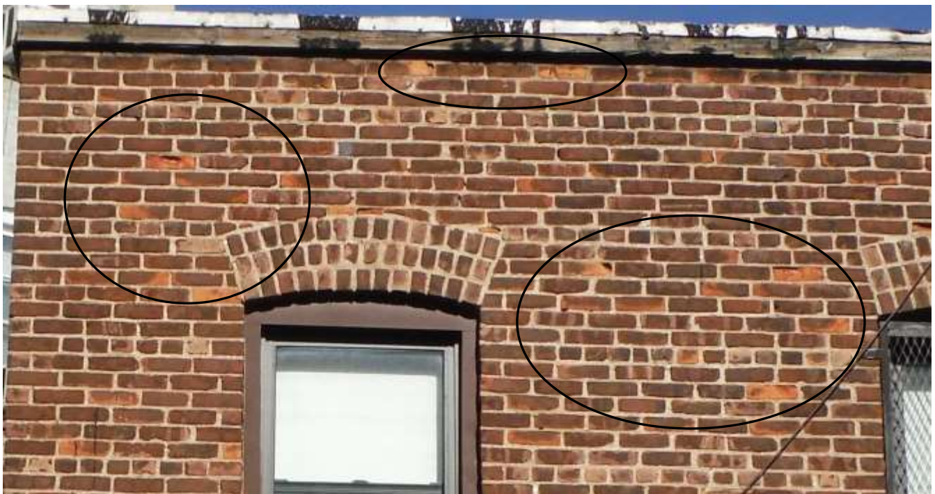
Figure 8 Brick damage; flaked, chipped, delaminated, water damage, efflorescence, cracks, etc.
