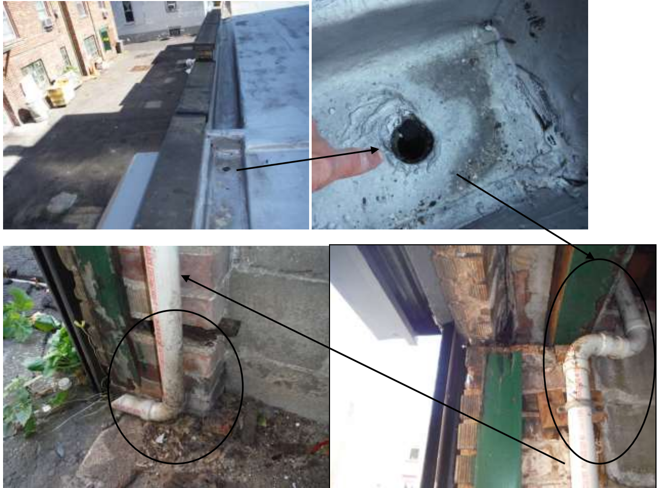
Figure 16 There was water damage to structure (walls, columns, roof sheathing) and a small PVC pipe installed from roof into garage and out the bottom of door. The drainage is too small/inadequate and handyman installation.
