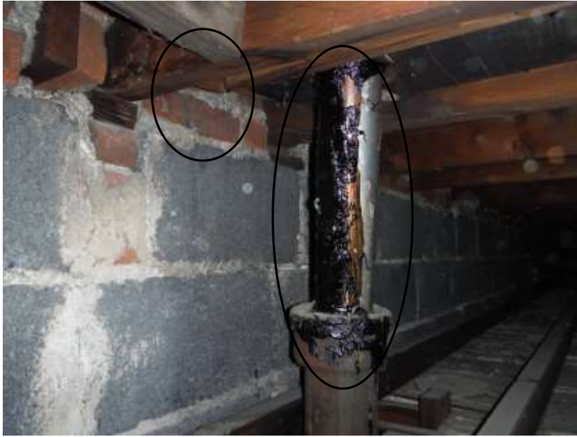
Figure 26 Cracks, splits, water rot, tarring, active leaks, etc. Have a roofer evaluate roof structure & advise on all roof and structural repairs.
