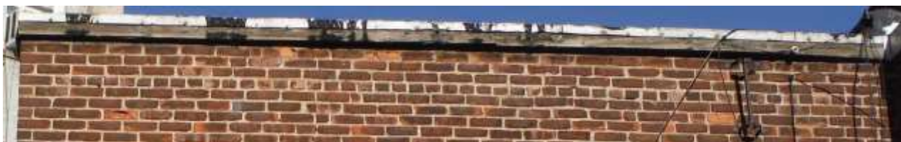
Figure 6 Exposed wood trim on top of building; have contractor evaluate/repair.
