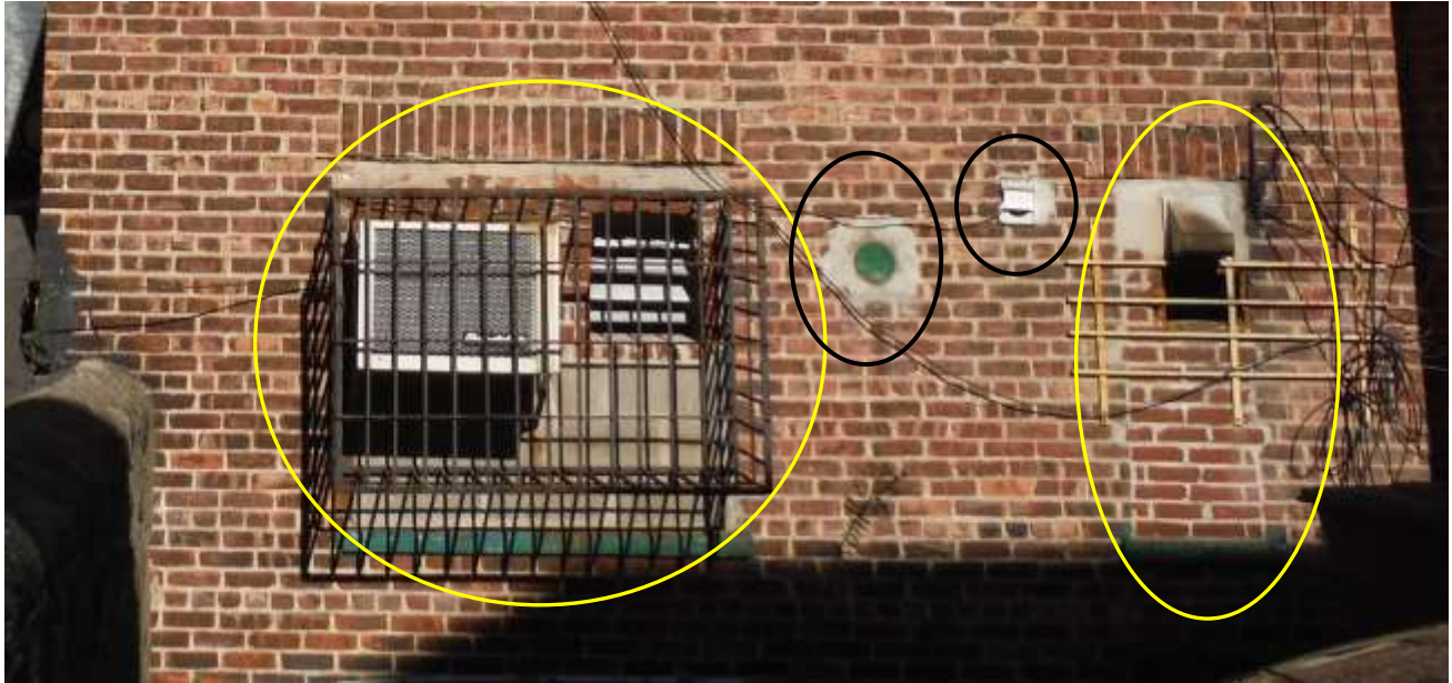
Figure 7 Two windows in rear were modified to make room for an A/C through wall unit and a vent. The right window was bricked up and a vent installed. Have a contractor seal up all open holes, remove old vents/blowers/abandoned equipment and replace broken vents where still in use.
