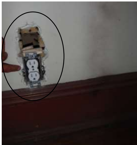
Figure 22 Example of electrical hazards in home.
